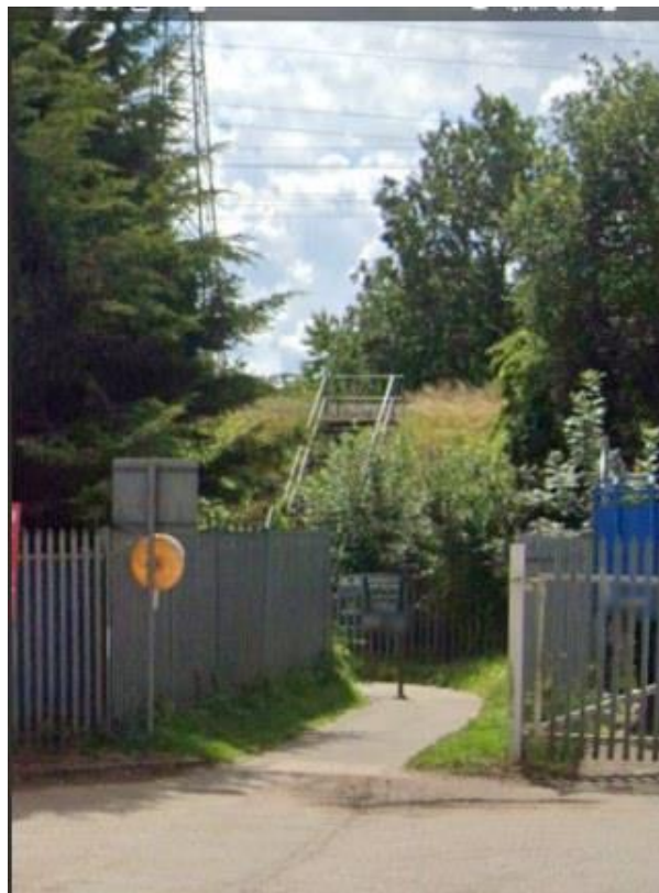
1 - Poor state of repair
